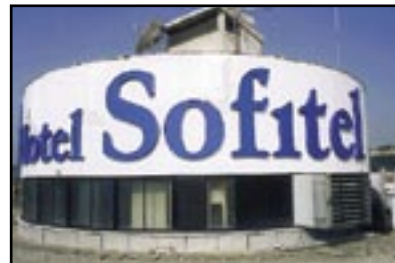
Base station blended into building facade
