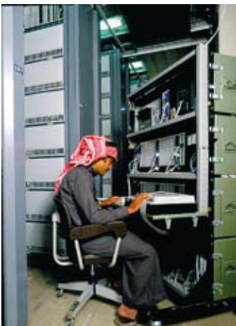
Figure 1 AXE telephone station, Saudi Arabia, 1978.
