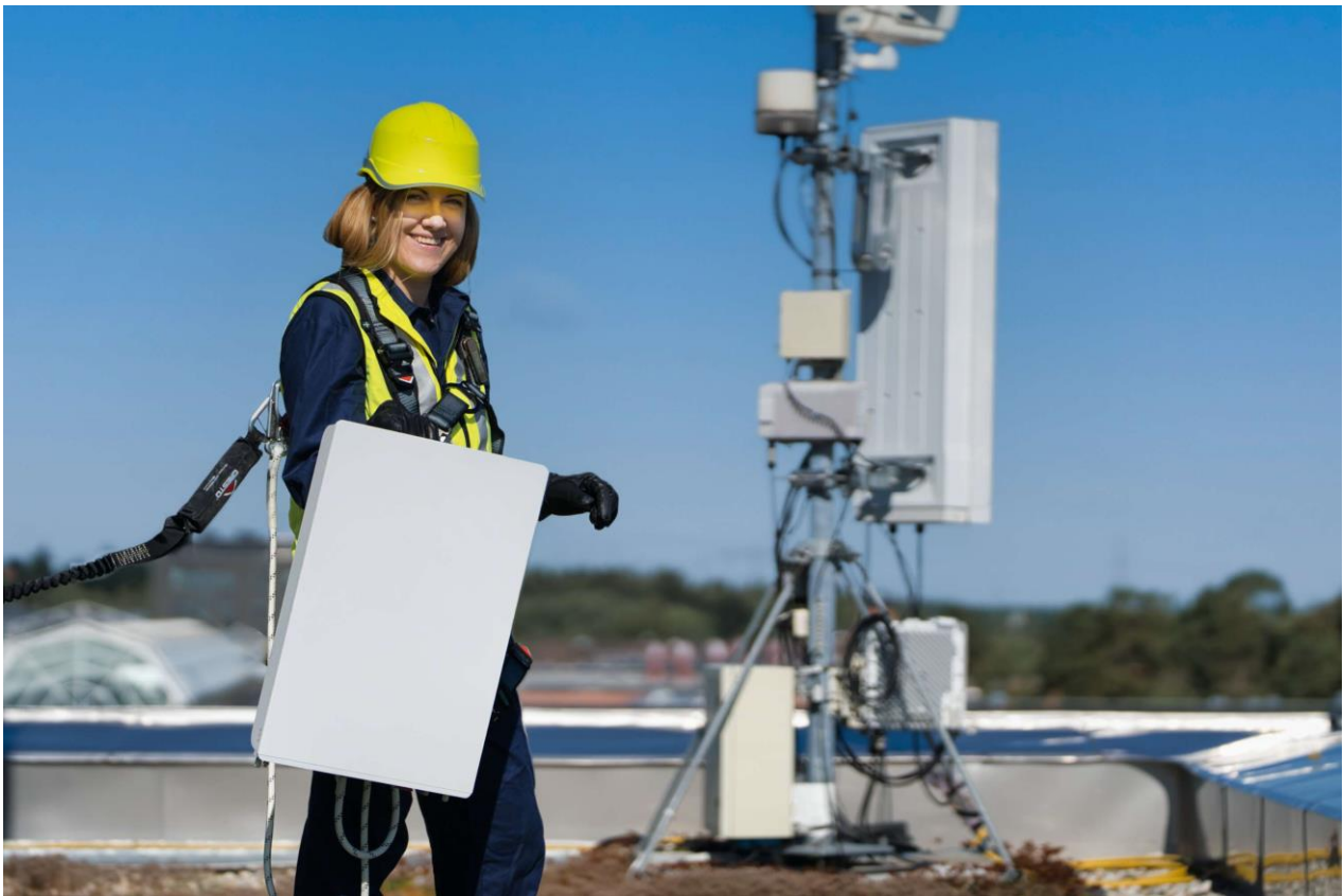
Ericsson Air 3268 radio rollout on a rooftop.
