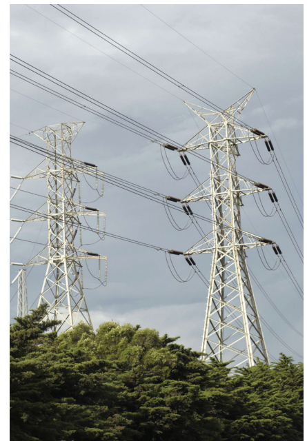
Network mechanisms are important for locating, identifying and fixing faults
