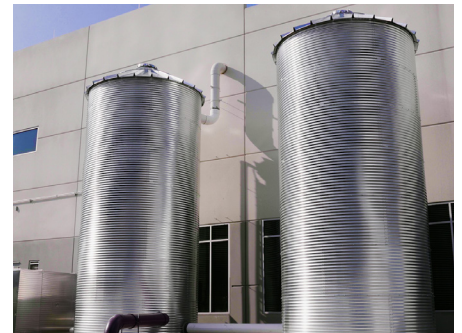
40,000-gallon water tanks collect, treat and use rainwater at the factory
