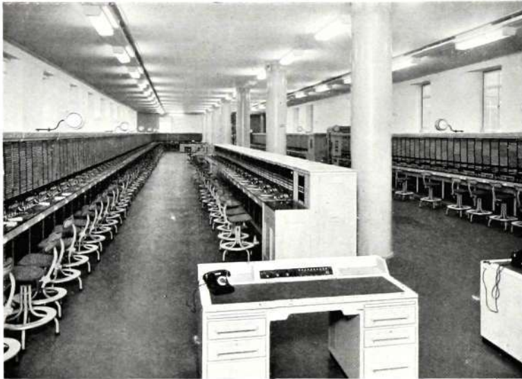
Fig. 7—The Manual Switchroom
