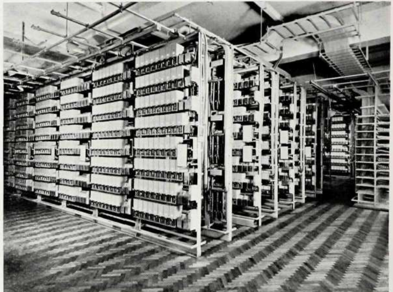
Fig. 5—Third Selector Racks. First Floor
