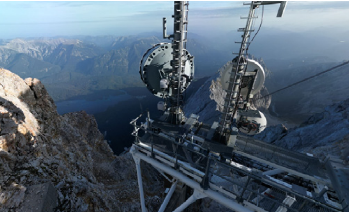
Harsh environments present significant maintenance challenges.
