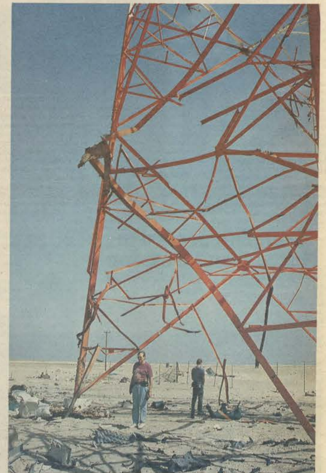
▲ This is the base for a 100-meter high radio link tower at the Salmi 1 site, which was bombed during the war. The majority of the base stations in Kuwait City stayed intact, but in the rest of the country some 90 percent has been destroyed. The old sites where the base stations were could perhaps be used again, but transmission networks have to be built up from scratch. In that case it will replace Kuwait's earlier mobile telephone network, which was a Japanese NEC network. But the NEC equipment was carried off by the Iraqis, who just have NEC switches. Ericsson's installed equipment on the other hand seemed uninteresting to them and was left intact - rather fortunately.
