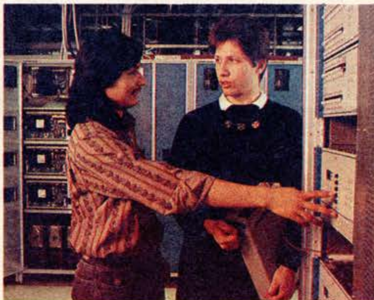
Current supply for telephone exchanges is becoming a more and more sophisticated affair. Power and telephony go hand in hand and work in close harmony. Expertise in power supply exists at Ericsson Components Power division in Kungens Kurva. In the picture Fernando Ruiz and Mats.
