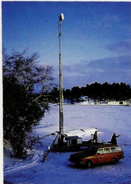
Fig. 12 A temporary MINI-LINK installation using a telescopic mast
