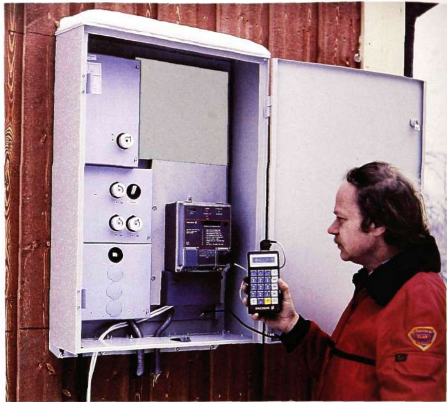
Fig. 7 Reading a meter installed outdoors in a cabinet
