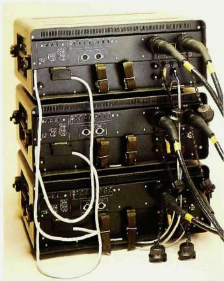
Fig. 4 All external connections and interconnections are made at the rear of the exchange
