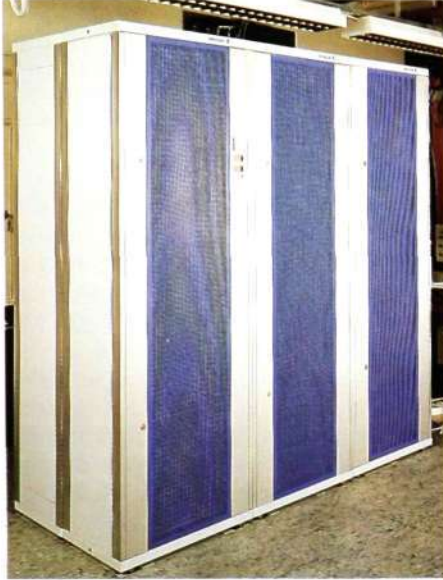
Fig 10 Power supply equipment BZA 204 05. The front row contains three cabinets with power equipment. The rear row consists of battery cabinets mounted back to back with the power cabinets
