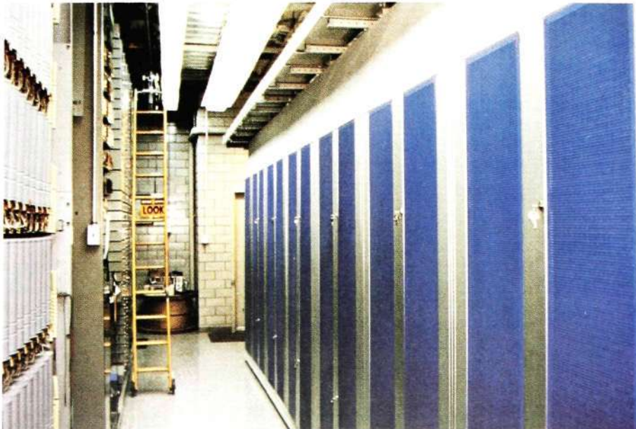
Fig. 5 The AXE 10 exchange installed on the same premises as the earlier step-by-step exchange
