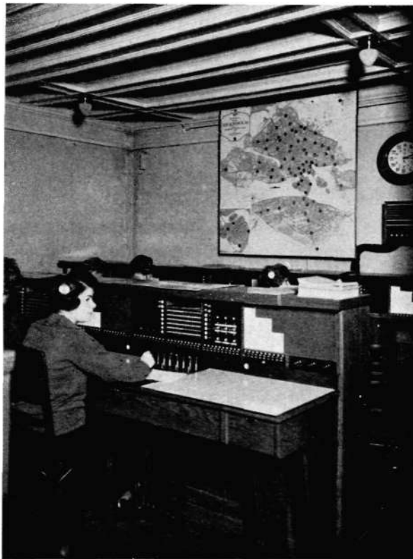
R 203 Fig. 1. Partial View of the Stockholm Taxi Telephone Exchange. Map with Indicator Lamps in the Background.
