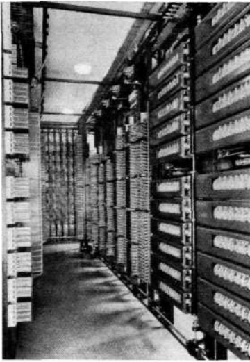
Fig. 3 Unit racks 1 and 2
