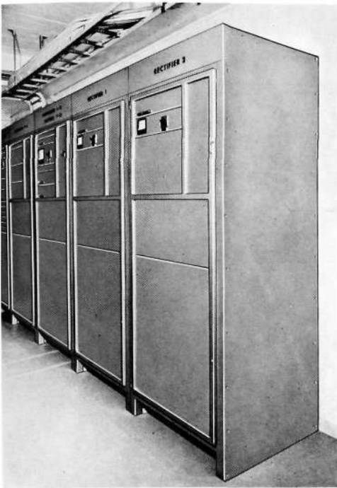
Fig. 10 Power supply equipment for 48 V with two 400 A thyristor-controlled rectifiers type BMT 173, two 400 A series converters type BMR 110 and one 1200 A distribution rack type BMG 201
