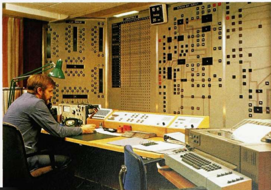
Fig. 2 A large part of the Swedish trunk network is supervised from the Swedish Telecommunications Administration's traffic supervision centre in Stockholm. Remote switching of lines and rerouting of traffic can also be carried out. The centre contains a test desk, which is remotely connected to the AKE 13 exchange in Hammarby (Stockholm). From here measurements and traffic observations are carried out on trunk and international lines. The lines are connected up to the test desk by means of commands on a remotely connected typewriter, which can also be used for other orders and printouts concerning the AKE
