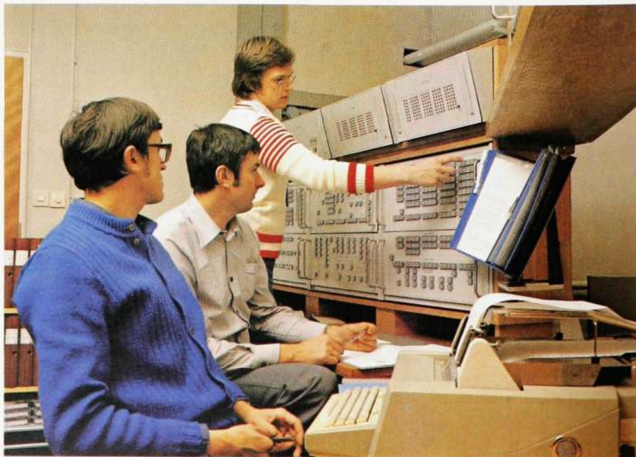
Fig. 1 LM Ericsson carries out extensive training activities with, among others, participants from the operating staff of the telecommunications administrations. Special AKE 13 exchanges with complete control rooms have been built up in Stockholm for training purposes. The picture shows one of these control rooms where two engineers from PTT in Czechoslovakia receive tuition in operation and maintenance
