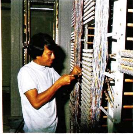
Fig. 7 Wiring of a rack
