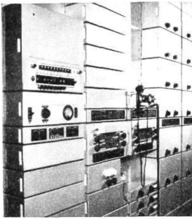
Fig. 16 Section of the Mariehamn exchange equipment
