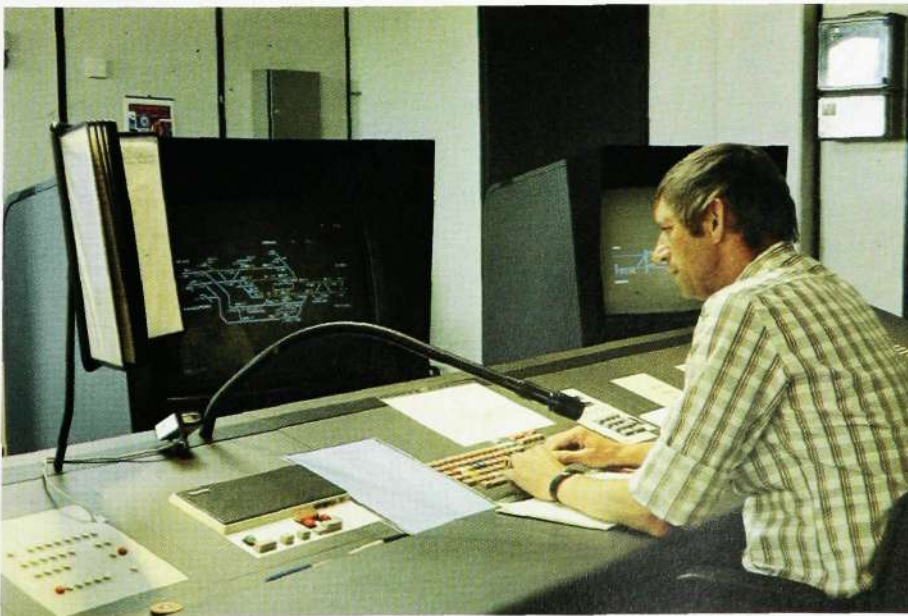
Fig. 11 Herning is equipped for two control positions. One is used for local control of Herning station. The other position is used for remote control of Holstebro station
