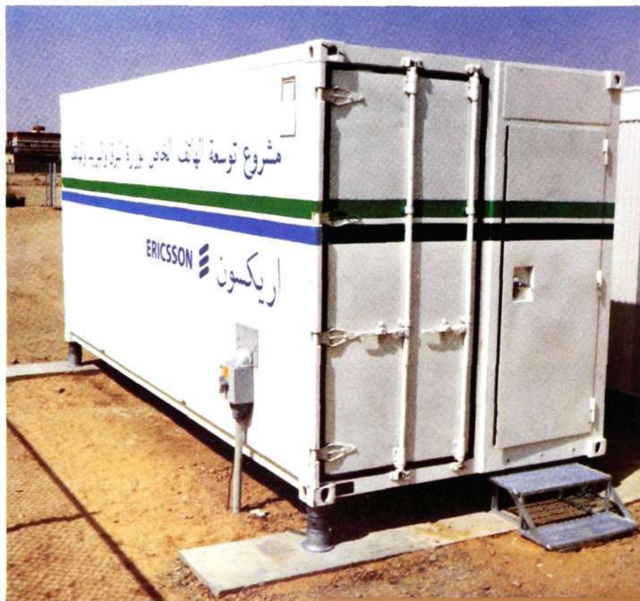
Fig. 1 A container in place and connected to the network in Saudi-Arabia
