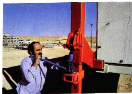
Fig. 6 Jacks are used at the installation site to lower the container onto its base
