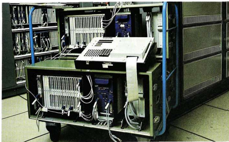
Fig. 6 Data traffic generators are among the aids used during the installation testing of the data network system
