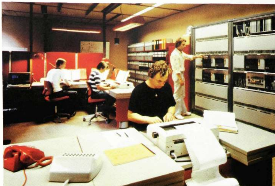
Fig. 11 The control room in the AXE 10 exchange at Ulriksdal near Stockholm when the exchange was being put into operation.
