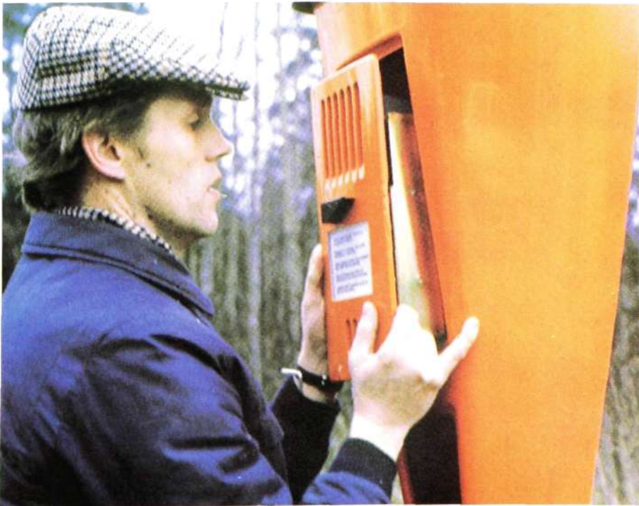
Fig. 5 The telephone cassettes are easily replaced, which simplifies fault clearing. The individual settings that specify the identity of the emergency telephone are made in the connection unit and are not affected when a cassette is changed
