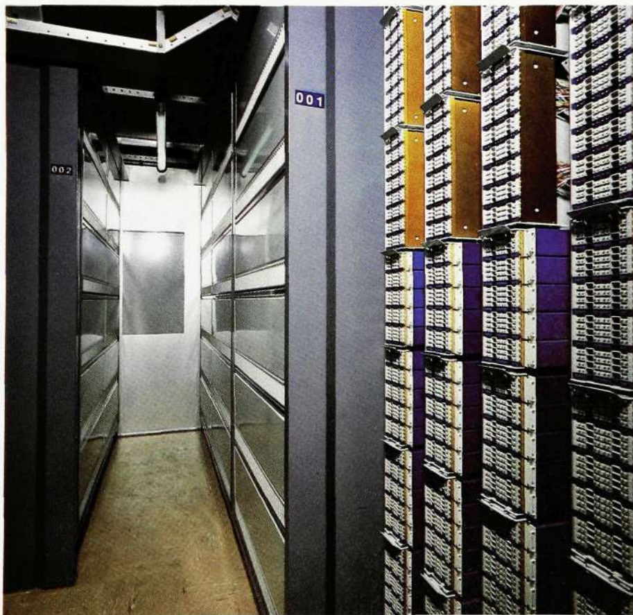
Fig. 7 Interior view of a container with equipment for 2048 subscribers. The main distribution frame can be seen in the foreground
