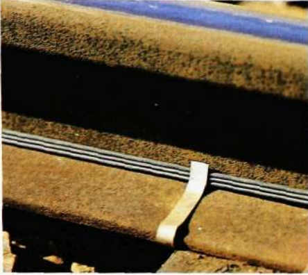
Fig. 8 A bracket holds the cable in place
