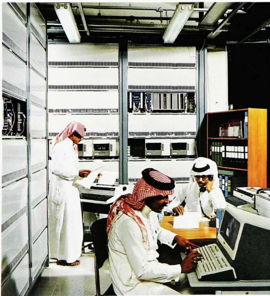
Fig. 8 Great emphasis was placed on practical work in the operation and maintenance training
