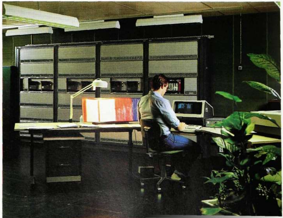
Fig. 1 The control room for AXB 30 at Hammarby, Stockholm, Sweden. Almost all operation and maintenance activities can be carried out from here
