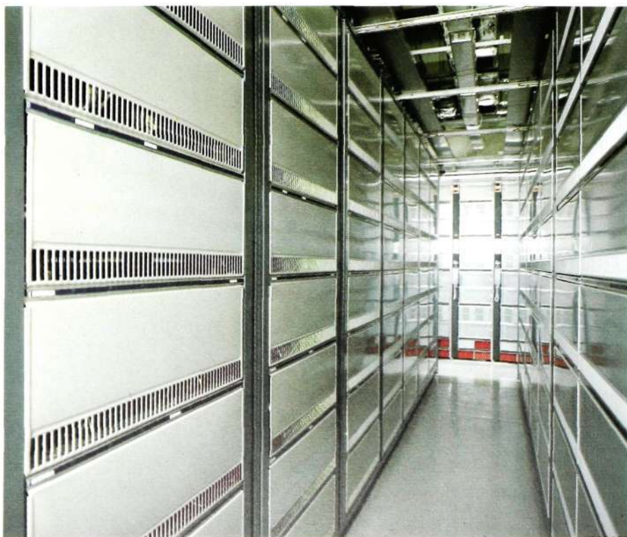
Fig. 1 The interior of an AXE 10 exchange
