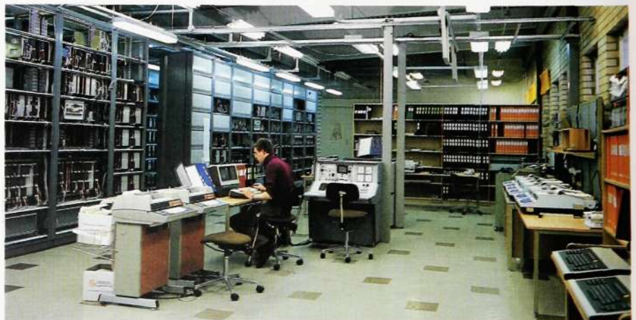
Fig. 3 The MIPSC unit dealing with the telex exchange systems, AXB 20
