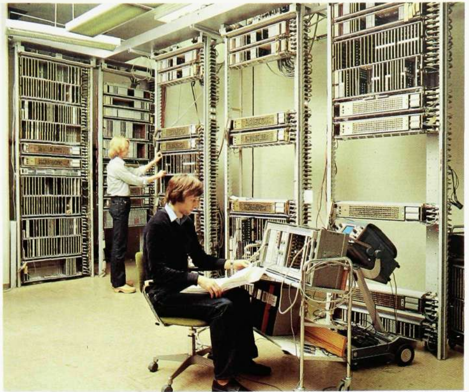
Fig.6 Work on toll ticketing equipment in the MIPSC unit dealing with the ARE systems
