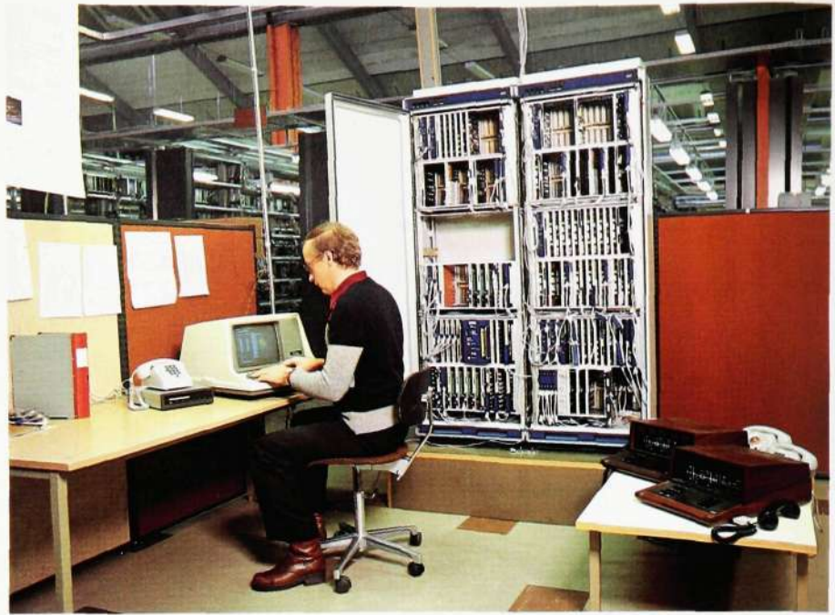
Fig. 11 PABX type ASB 900 installed in the MIPSC unit dealing with stored program controlled PABXs
