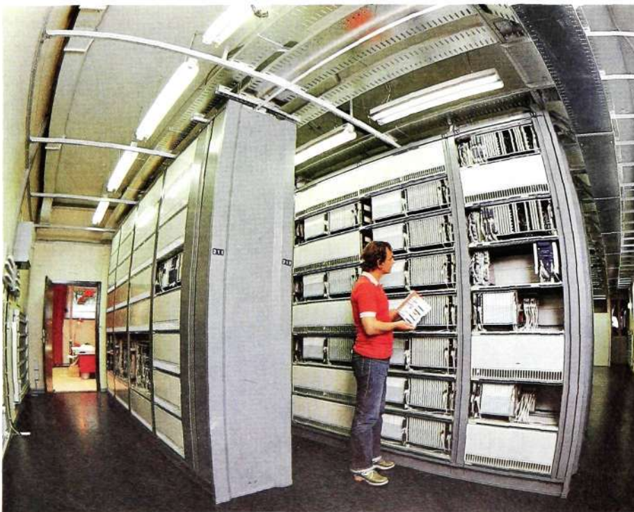
Fig. 12 The AXE 10 exchange at Ulriksdal, Stockholm, delivered by Teli in 1980
