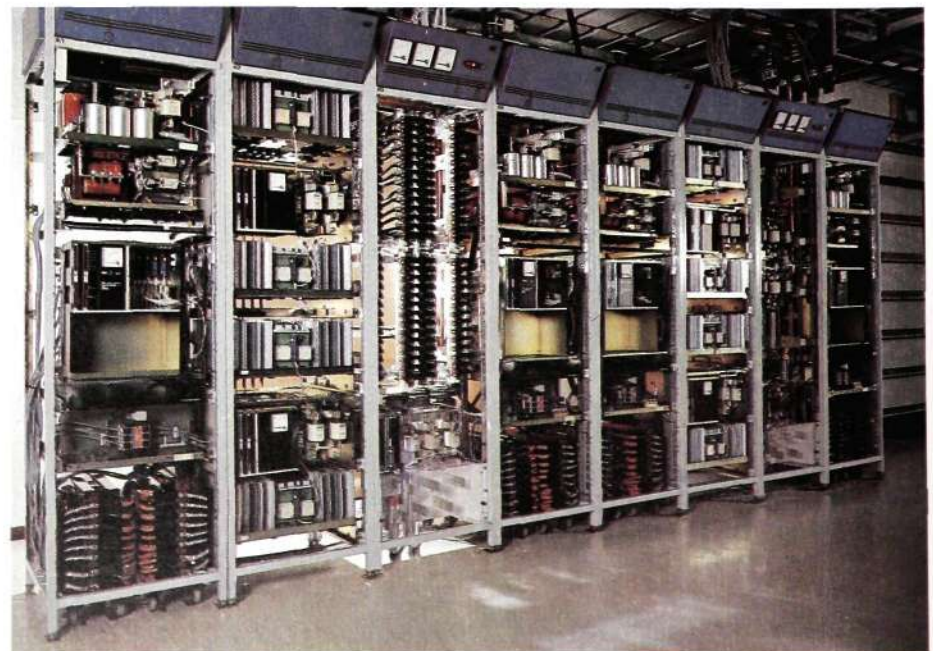
Fig. 14 The illustration shows two plant modules, each for 800 A, consisting of two rectifiers between which the converters and distribution have been placed to limit the current in the top bars
