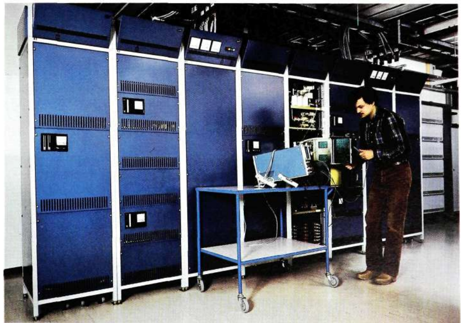
Fig. 1 Type testing the power supply plant BZD 412 in the laboratory
