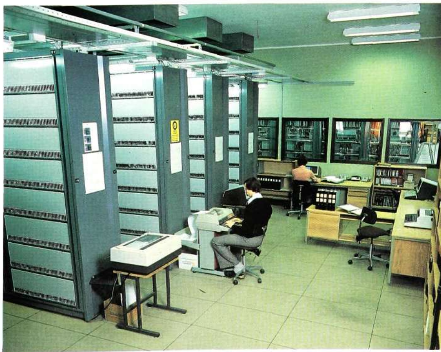
Fig. 2 LM Ericsson have established a Maintenance, Installation and Production Support Centre, MIPSC, in Stockholm. The picture shows an AXE 10 exchange in MIPSC. It is employed for detailed analysis of complex problems
