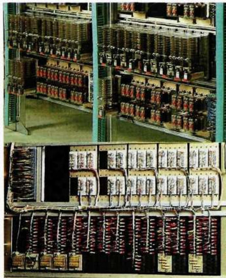
Fig. 1 The degree of safety obtained with robust relays, large insulation distances between the circuit elements, guided contacts and simple circuit structure corresponds to what is obtained with large information and system redundancy in a computer controlled system
