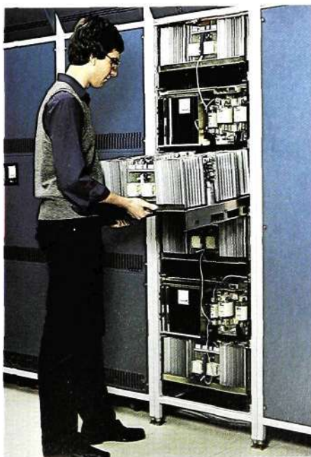
Fig. 15 The equipment consists of factory-assembled units which are slid into the rack on guide rails
