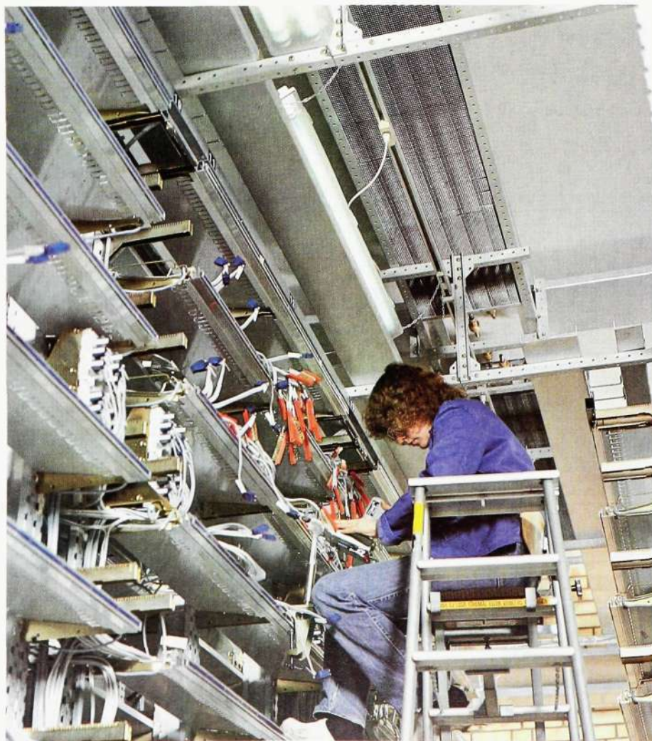
Fig. 8 The cooling coils are mounted above the aisles between the equipment suites
