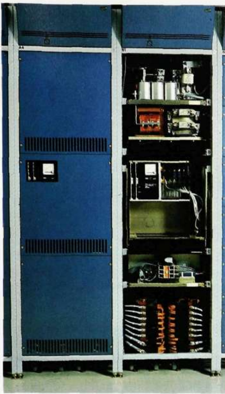
Fig. 4 Two thyristor rectifiers BMT 343, one with front panels and one without
