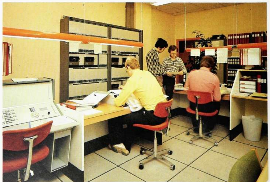
Fig. 3 The control room in the AXE 10 exchange at Södertälje, completed in 1977
