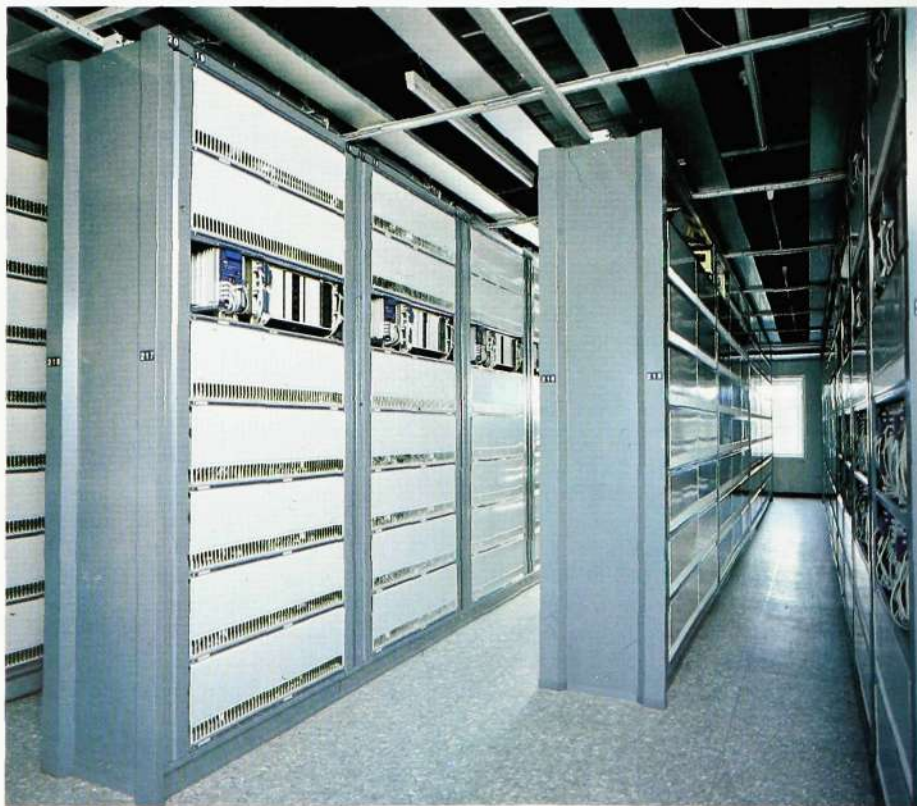
Fig. 1 A transit exchange in Kolding, Denmark, for 8000 junction lines
