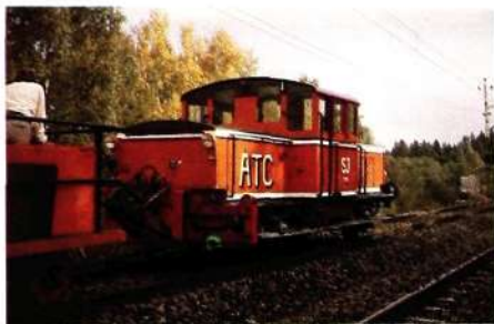
Fig. 15 Installation. The Swedish State Railways have made great efforts to get the ATC system installed and taken into service as quickly as possible. Several aids have been developed to simplify the installation in the track. The picture shows one of the three special vehicles that plough down the cables which connect the encoders and the beacons
