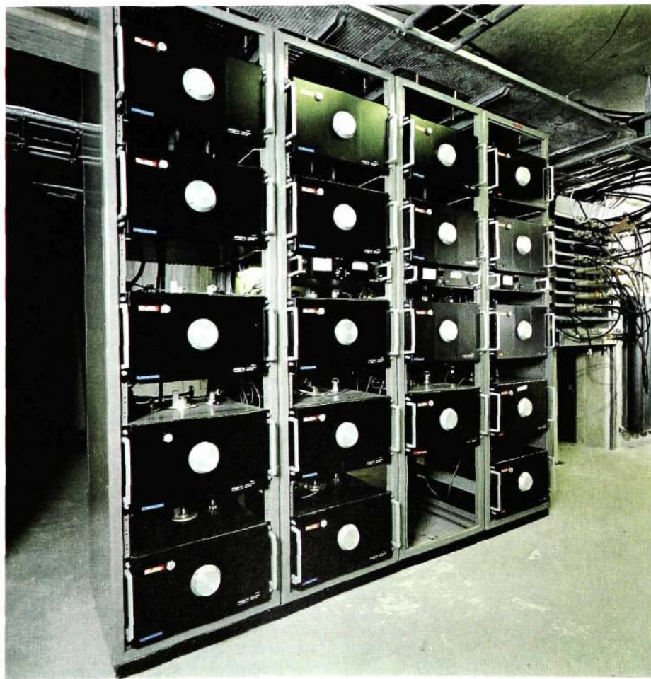
Fig. 5 Equipment for combining a maximum of ten channels to a common output or antenna. The picture shows one unit for ten channels and one for nine.
