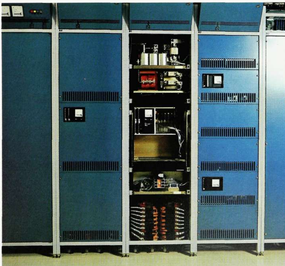
Fig. 1 Power supply system BZD 412. The picture shows, from the left, distribution rack BMG 651, a rectifier BMT 343 with front cover, a rectifier without the front cover and two 400 A converters, BMR 273. Each rack has the dimensions 600×600×2200 mm
