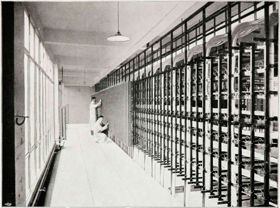
The Paris Telephone Exchange, France. Cross Connecting Frames
