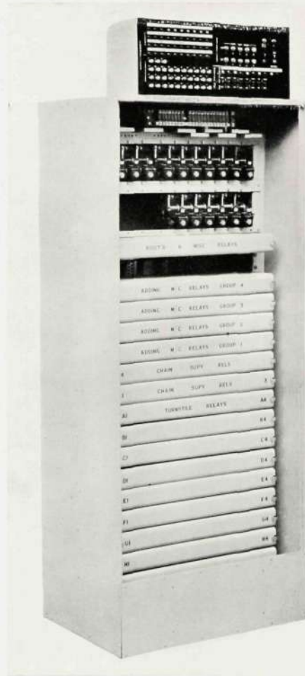
Fig. 2.—Attendance Aggregator Main Equipment Rack
