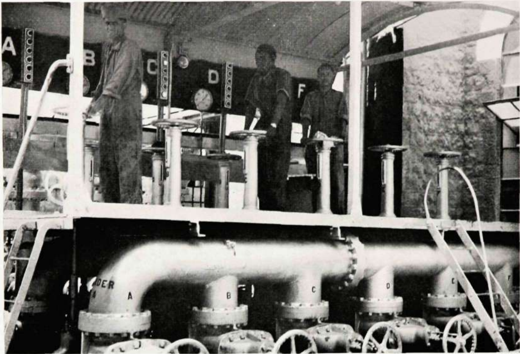
Fig. 6—Oil Control Valves
