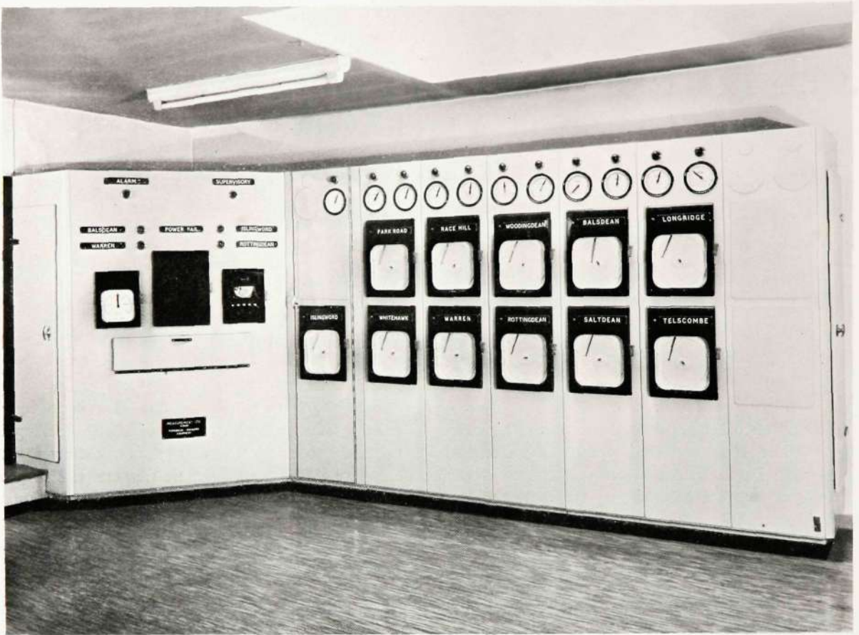
Fig. 1—Typical Water Supply Control and Indicating and Recording Equipment Panels
