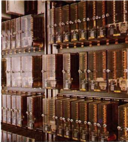
Fig. 18 Plug-in safety relays are still predominant in interlocking systems not using "geographical" system as in fig. 9
