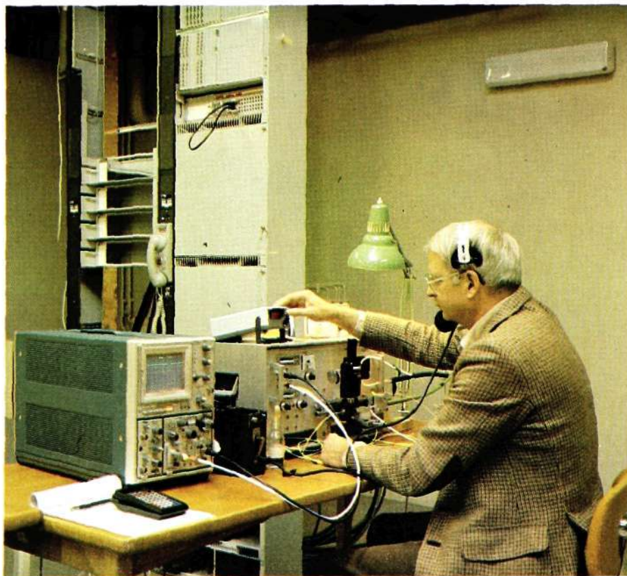
Fig. 8 Measuring station for fibre cables in the Fredhäll exchange
