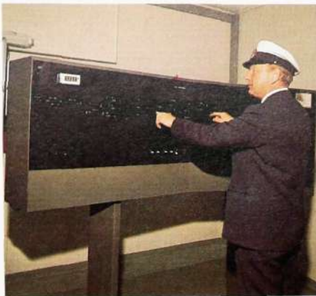
Fig. 14 In stations with local interlocking control the signals may be set with keys in the track diagram
