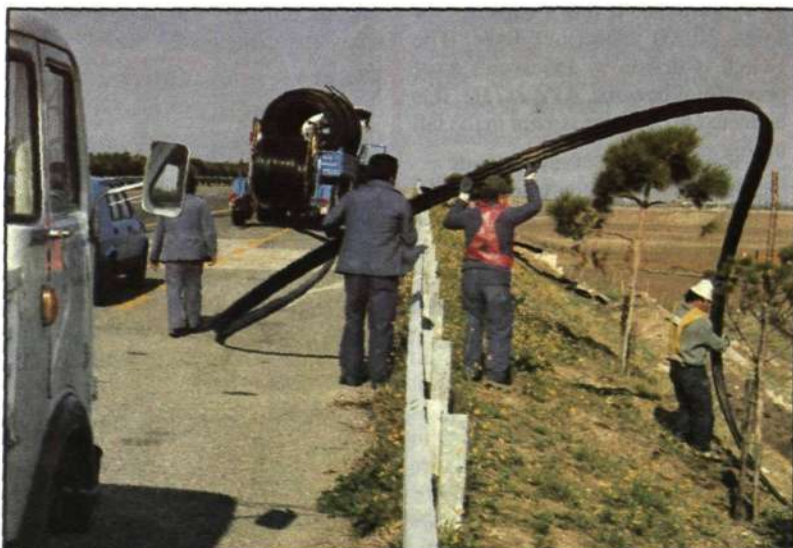
Plastic canalization piping is of Sielte's own construction and is manufactured by EL.TE. in Sicily.
