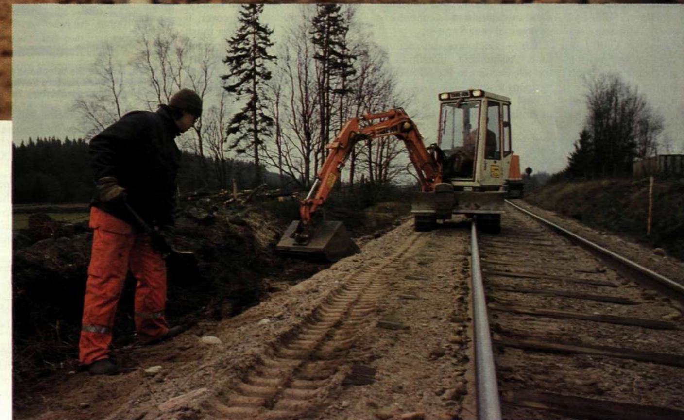
Refilling and cleaning up after cable plowing, with Janne Karlsson at the shovel.
