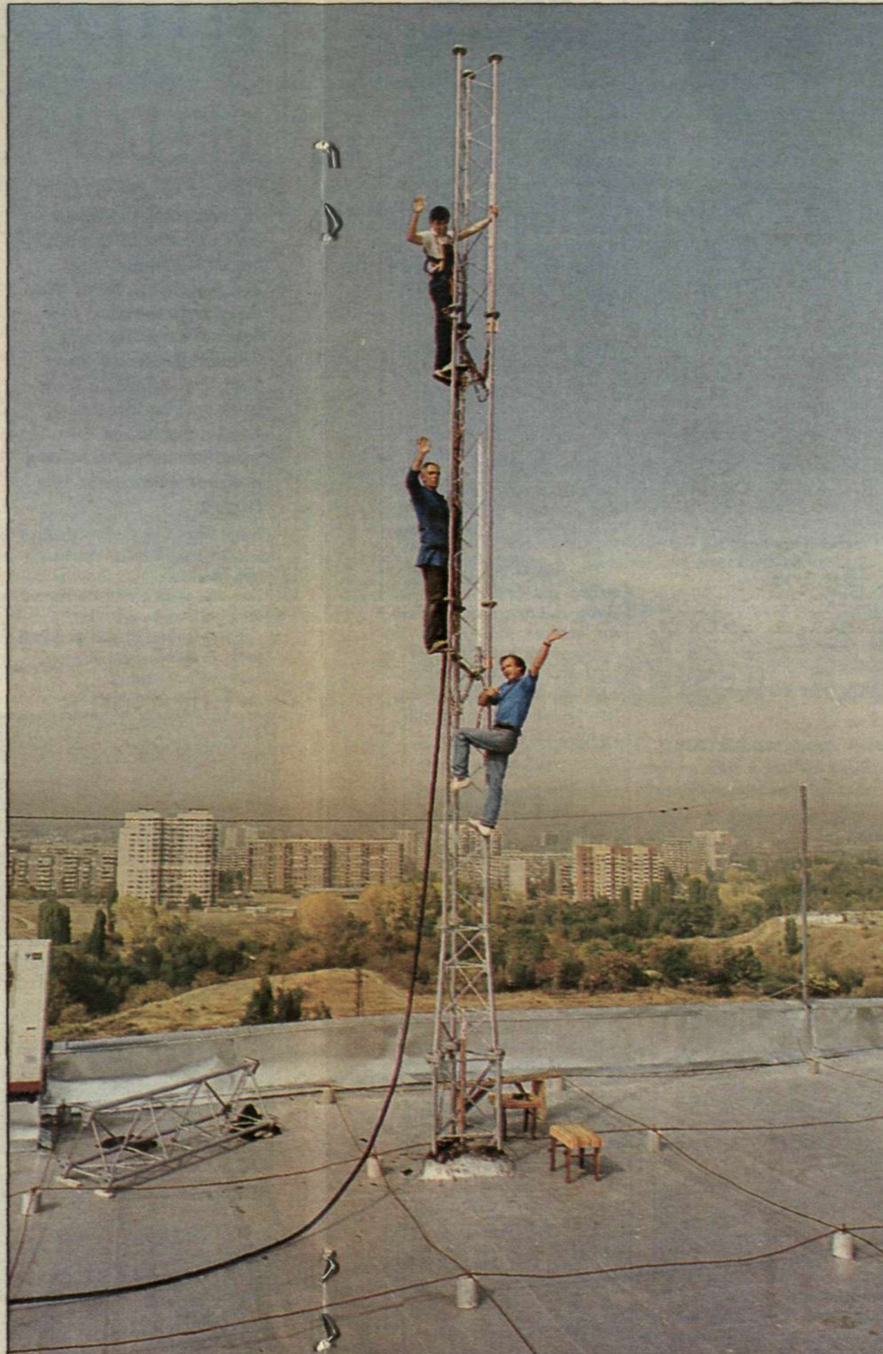
WITH EYES SET ON THE STARS. An NMT antenna being mounted at site 74 in Sofia. The picture was taken last October. At that time the network was being built up so as to be able to be put into operation already by Christmas.
