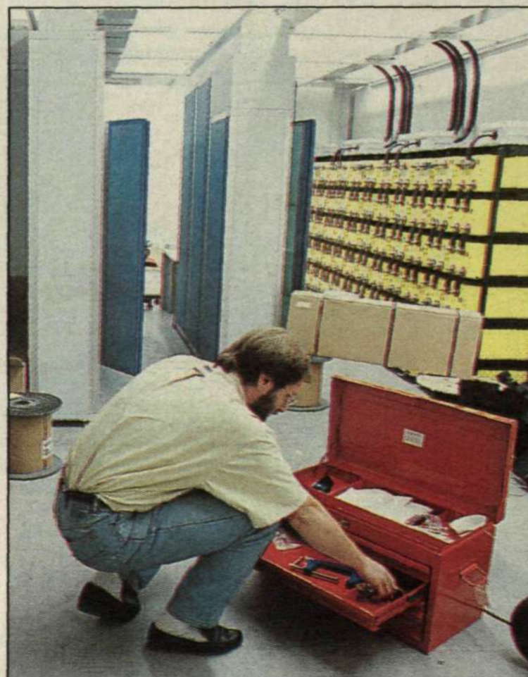
FULL SPEED AHEAD WITH EXPANSION. From inside the site in Sofia where Ericsson's switch was expanded upon at a fast pace for new channels in the mobile telephone system.
