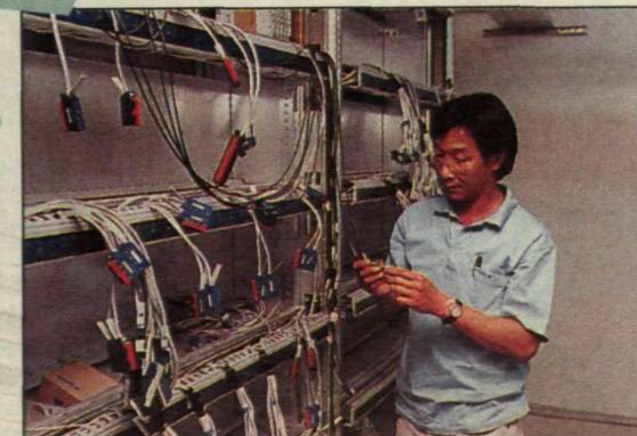
Installation of equipment at Telephone Organization of Thailand in Chiang Mai. Ericsson's largest Thai project involves installation of 500,000 new lines in the northern parts of the country.
