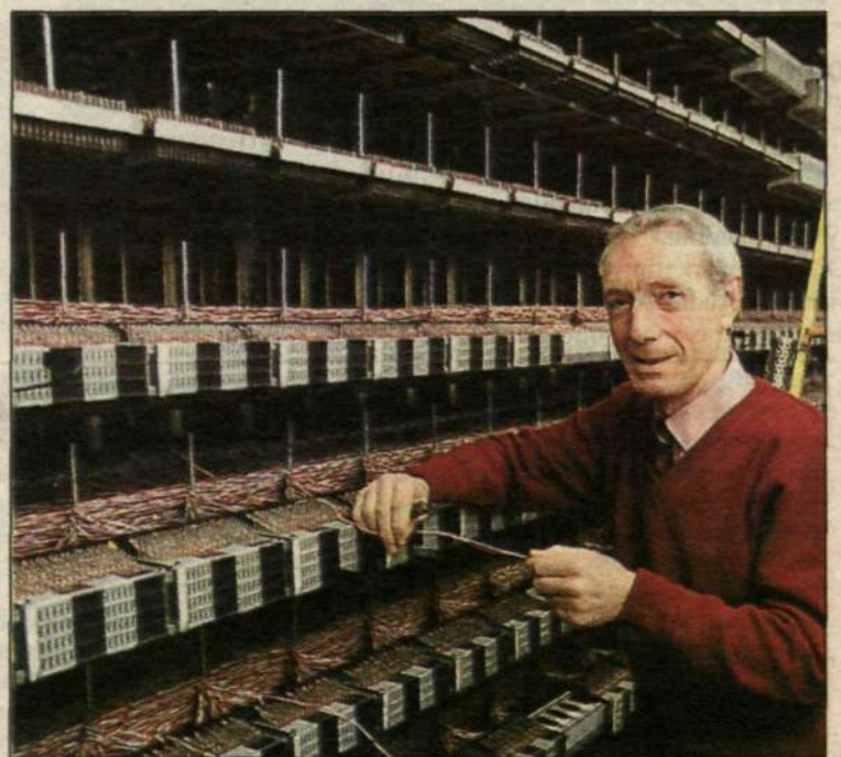
Barone Gildo, who recently turned 58, has worked as a telecom technician at SIP for 37 years. He is one of the many technicians who has been around since the 1950s, when Ericsson's first exchange was installed in Venice. "It seems like only yesterday that he began working, not half a life ago," says Barone.
