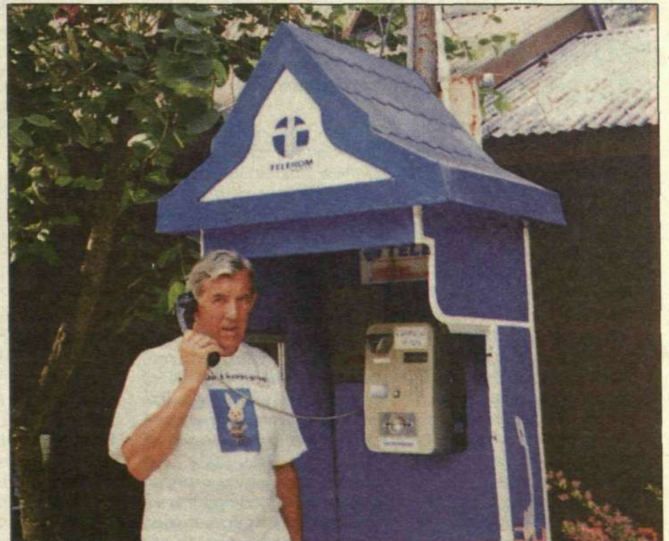
Hans Aronsson from Ericsson Radio Access places a call from one of the telephone booths served by the RAS 1000 system.
