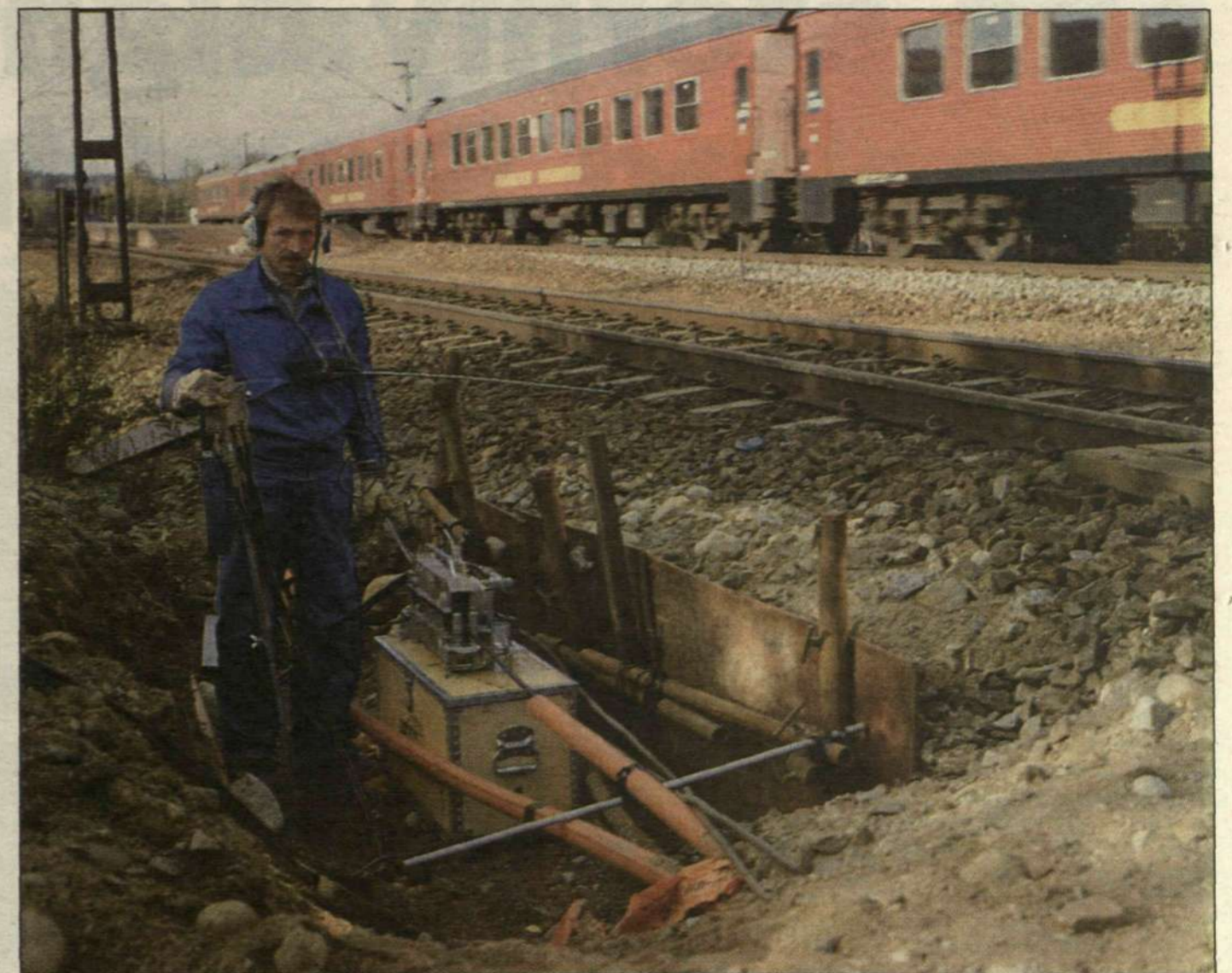
The Swedish State Rail Administration was very foresighted in laying fiber optic cable for its telecommunications network. Plans were made from the start to lease capacity to new telecom operators. Photo: Thord Andersson
