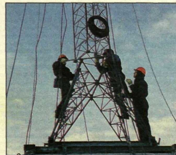
The exciting final seconds – when the mast is secured to its foundation. Ready for use!
