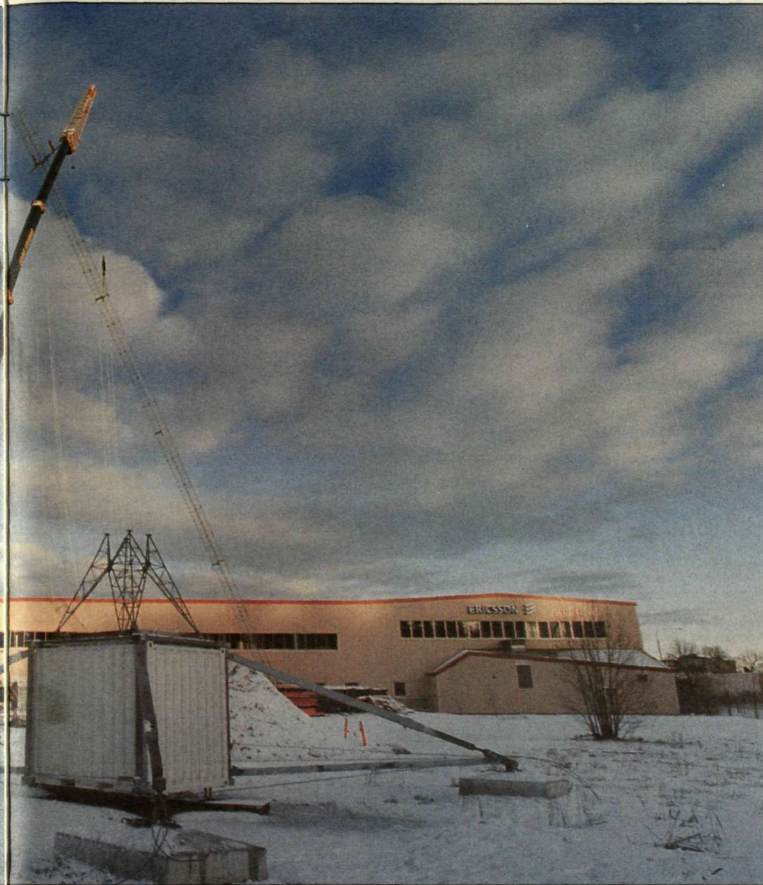
2.5-ton foundation plate. The entire station can be assembled by three men in two days, ready for erection by crane. Photo: Thord Andersson
