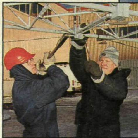
With experienced hands, Bengt-Åke Nilsson and Björn Aronsson check the tightness of all the nuts on the mast before it takes to the air.
