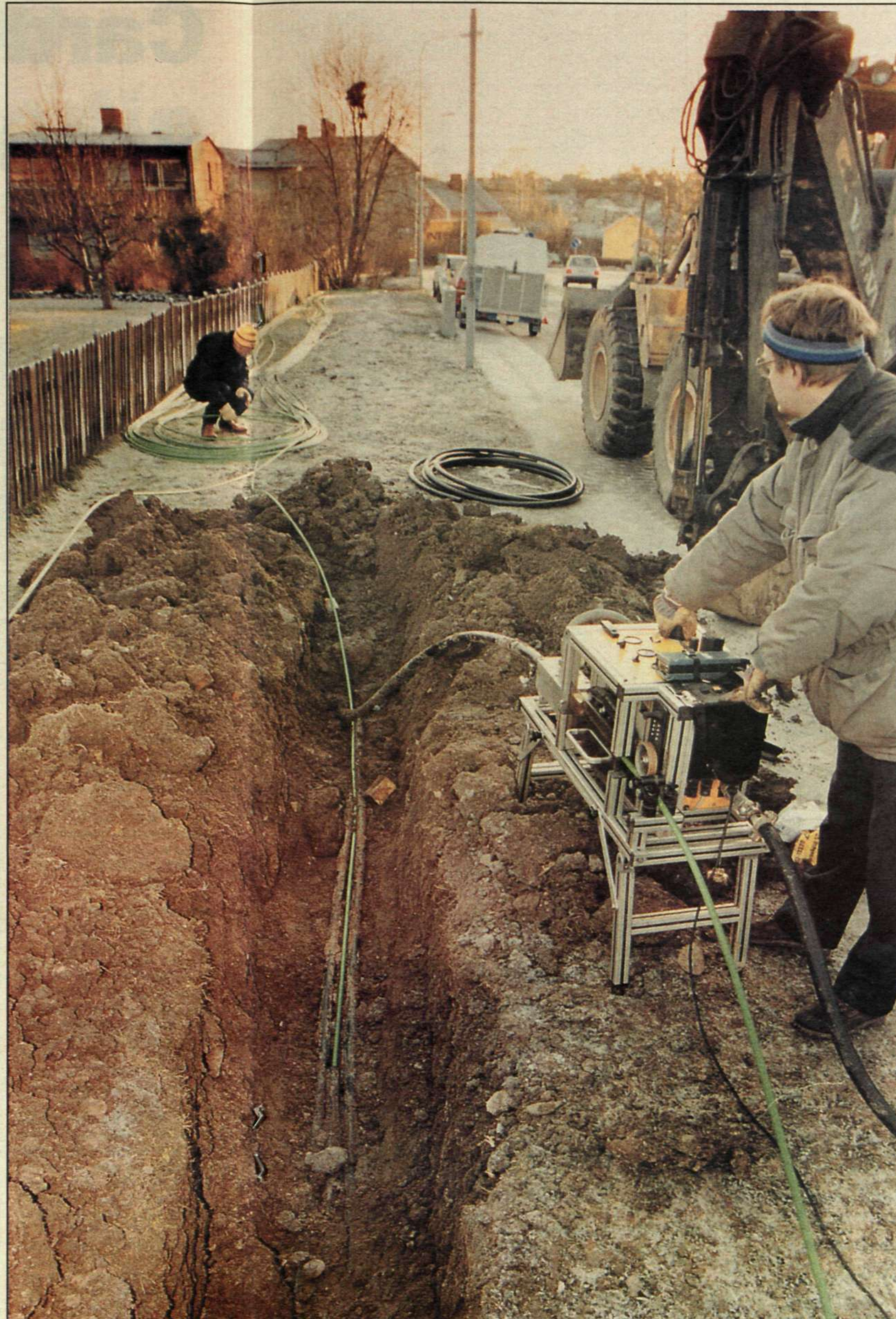
Hans Bjerneby with the new pressurized air machine from Lancier. Using 10 tons of pressure, he blows a 96-fiber cable into a pipe somewhere among the homes of Älvsjö.
