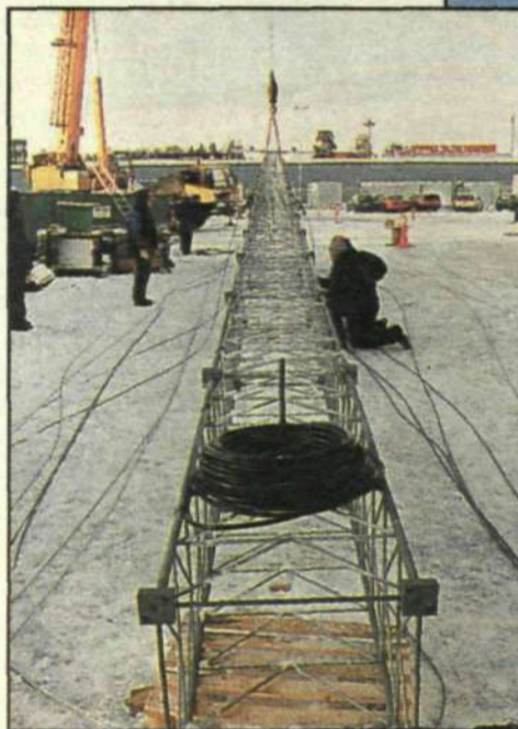
The Swesite mast is assembled and ready for erection. The mast consists of a number of 2-meter-long sections bolted together. Each section weighs 70 kg.
