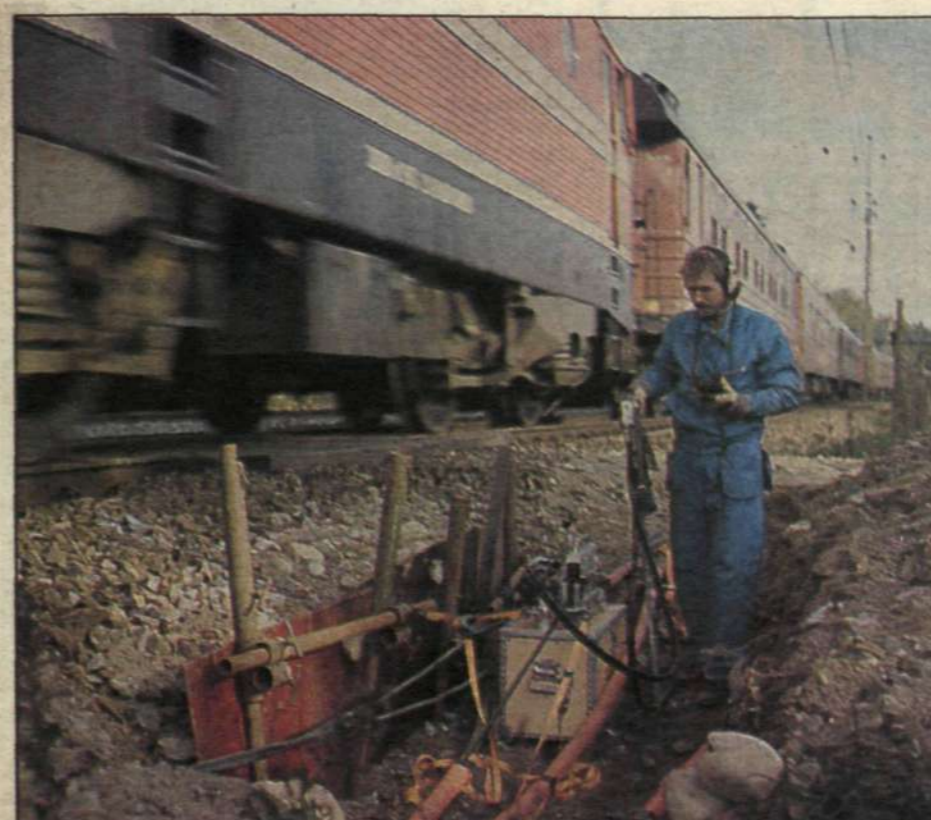
Many "new" companies are now focusing on becoming telecom operators. The Swedish State Rail Administration, which is leasing its new fiber optic network to Tele 2, among others, is a good example of a company without previous experience in telecommunications that now wants a share of the future market.
