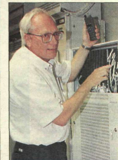
The World Championship exchanges were secure in the hands of Lars Cederquist, shown inspecting one of the ten MD110 LIMs which comprised the net group of 1,500 connections, which in turn were connected to the AXE network.
