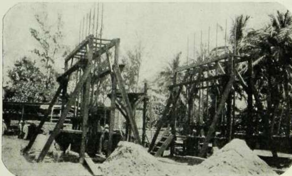
R 866 Placing a Coating of Asphalt on the Bases of Mannesmann Steel Poles for the Toll Line Between Mexico City and Vera Cruz.
