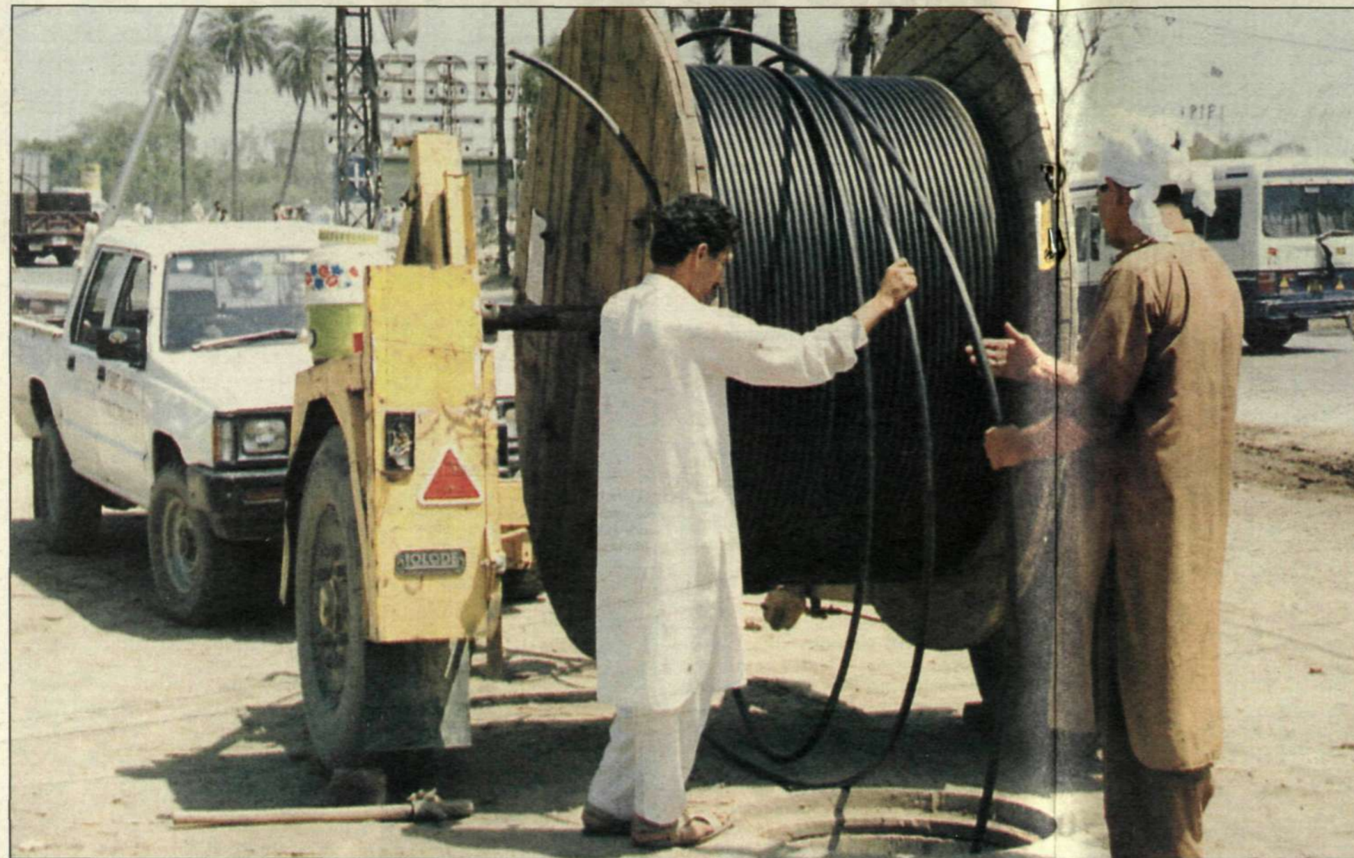
Cable is laid from one of the 4,000 cable drums required for the network installation project.
