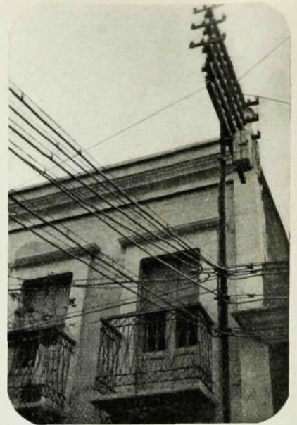
R 1019 Intake Pole near Exchange Building. The Bolivia Telephone Net.
