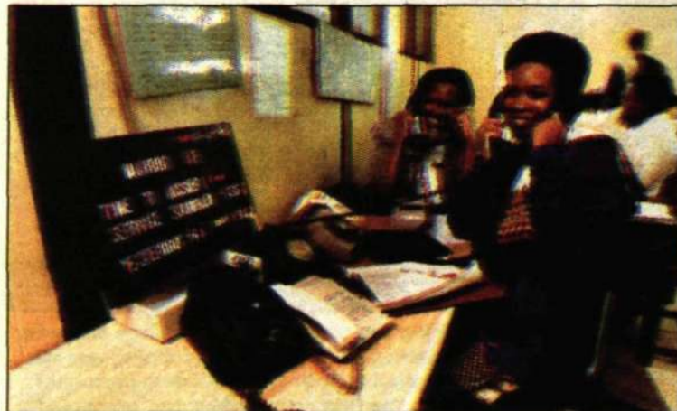
The telecom network in Kenya consists of a variety of equipment, ranging from manual switches to Ericsson AXE switches.
