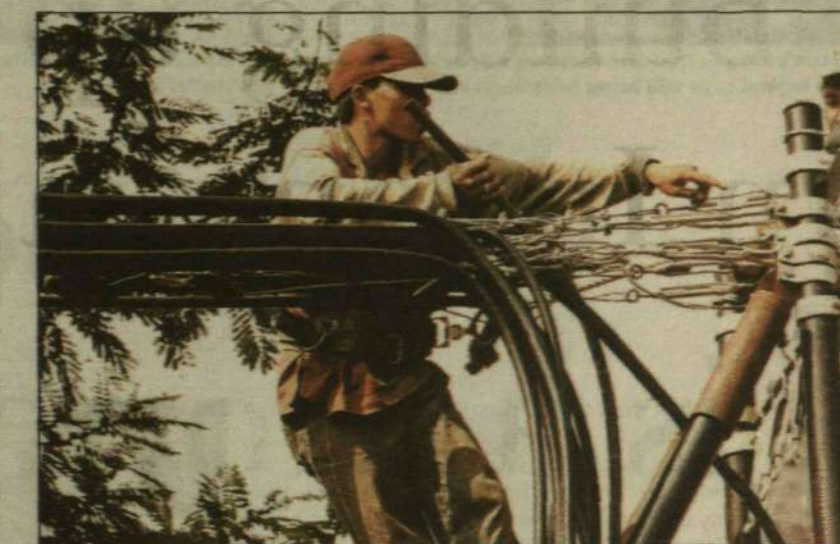
Indonesia is in great need of improved telecommunications. Bad roads and inaccessible terrain make a speedy development difficult.
