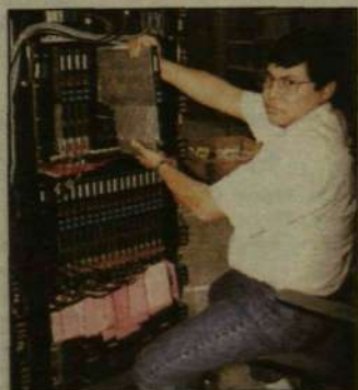
Paul Rivas holds up one of the transceivers on the 450 system channel tester.
