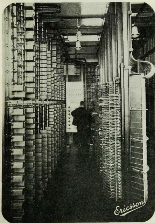
R 1039 Interior of the Telephone Exchange at Smyrna. Selector stand with the Switchboard in the background.
