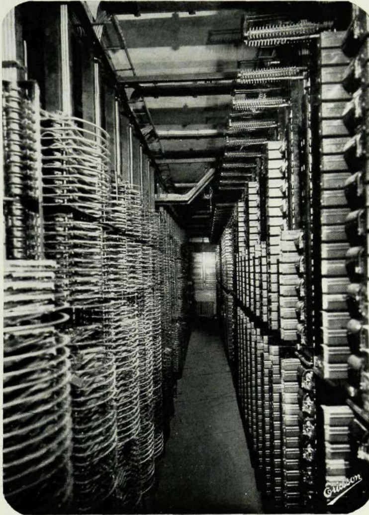
R 1075 Fig. 10. Interior of the »Borsa» Telephone Exchange.
