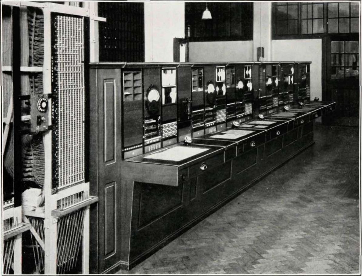
Hampstead Exchange—Test Jack Frame and Test Positions
