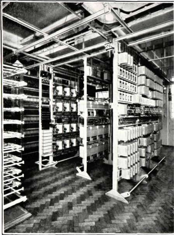
Hampstead Exchange—Coder and Sender Racks
