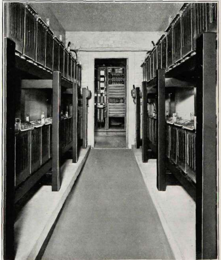
The Battery Room
