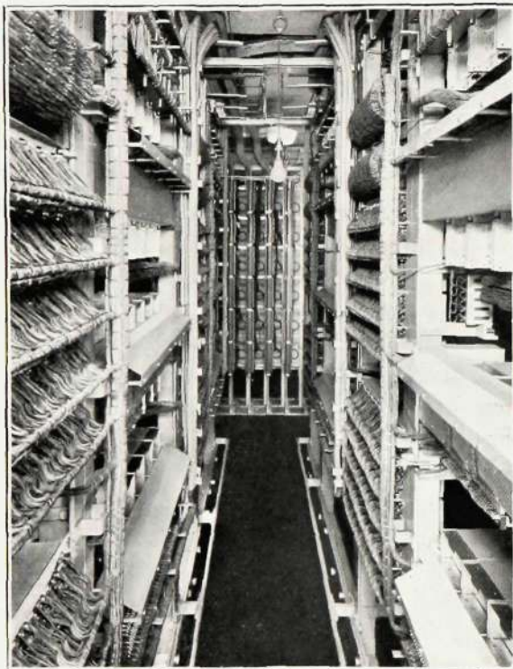
View between the Units with the Combined M.D.F. and I.D.F. in the background
