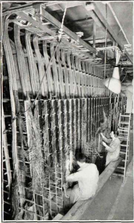
Fig. 3—Cabling and Wiring Multiple Side I.D.F.
