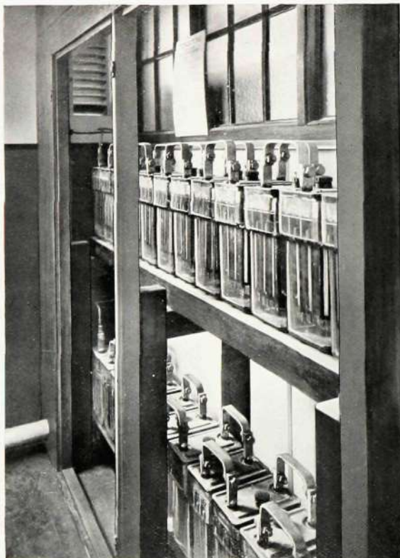
The Battery Room
