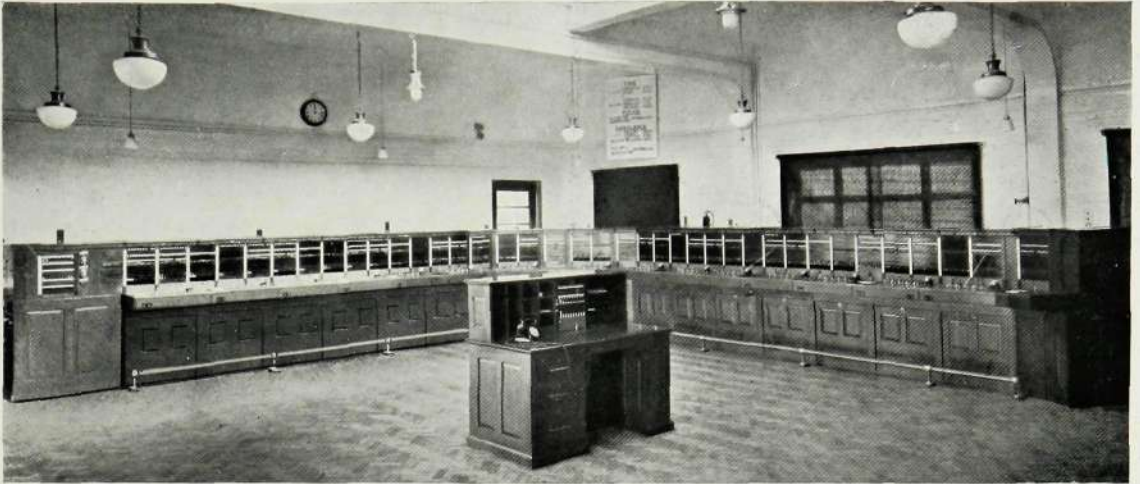
Fig. 8—The Manual Switchboard and Supervisor's Desk
