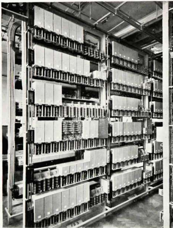
Fig. 6—Final Selector Racks
