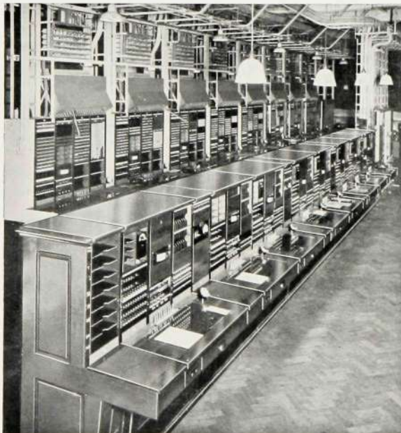
Fig. 2—Test Desks, Trunk Test Racks and Test Jack Frames
