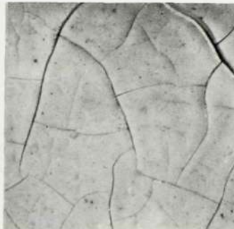
×8 Fig. 27—Paint Finish, Marked Deterioration.
