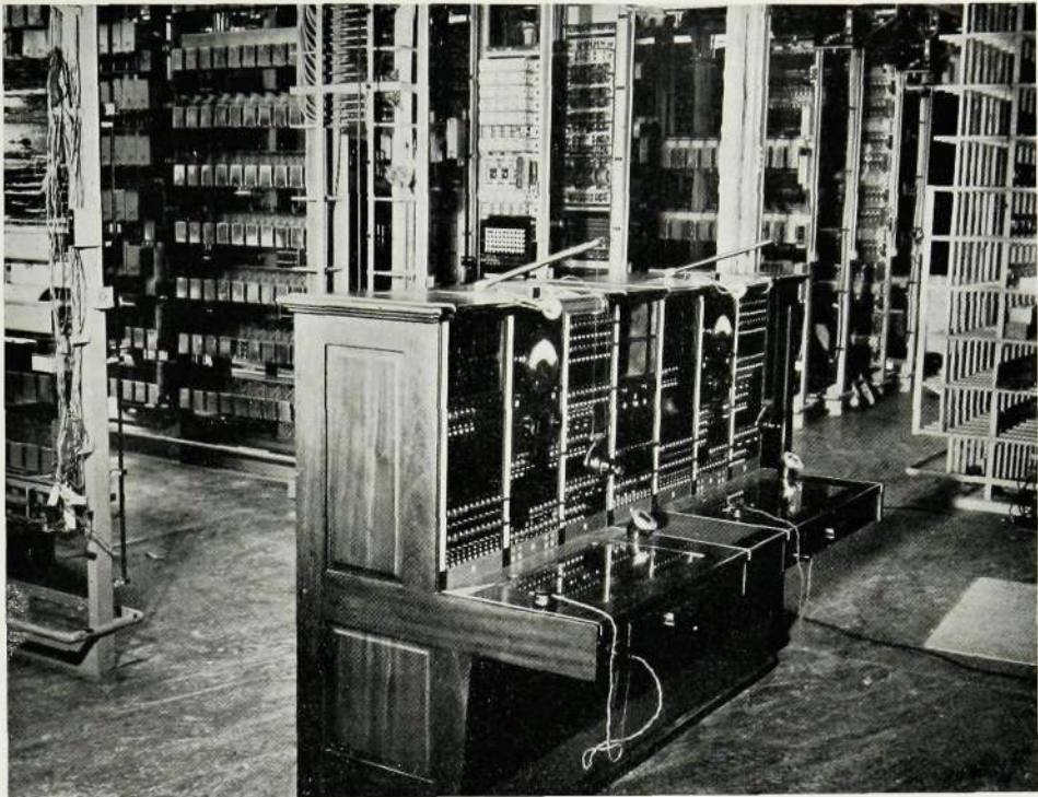
Fig. 3—Test Desk and Auto Equipment Racks during Installation.
