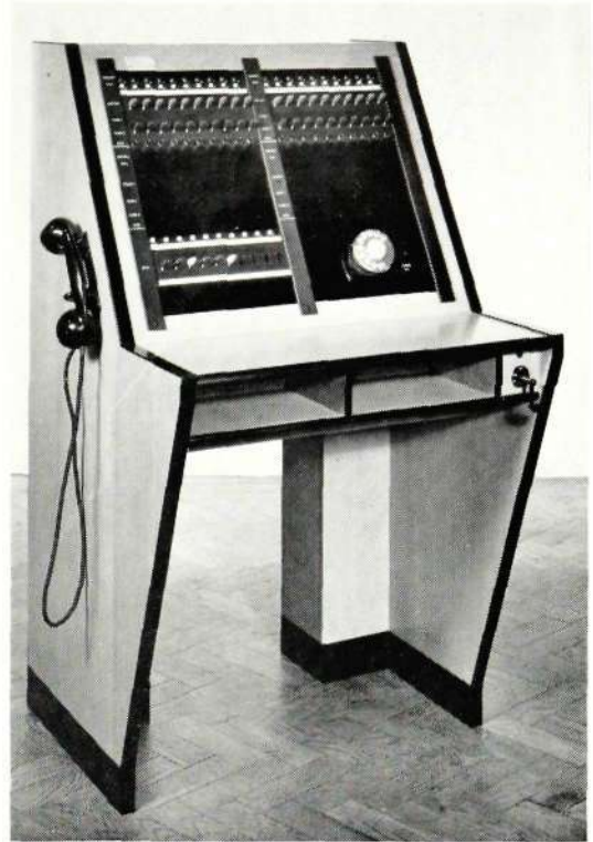
Figure 7—Mine emergency switchboard
