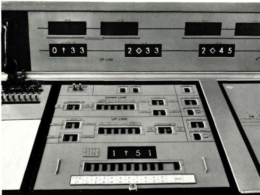
Figure 8—Fringe signal-box set-up panel equipped with a key for each character appearing in train description
