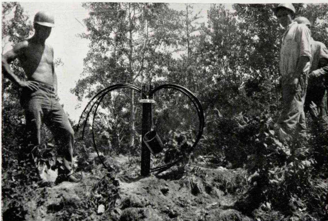
Figure 3—North American standard type cable post for connection of successive cable-drum lengths
