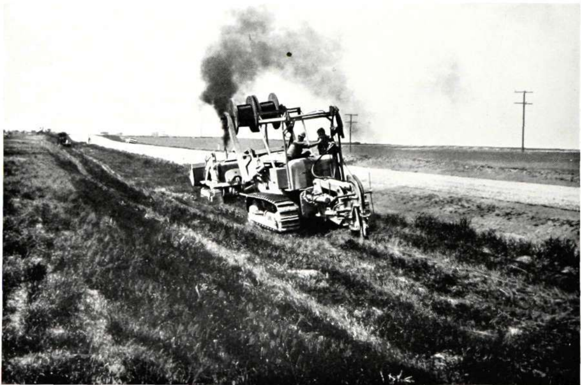
Figure 7—Ploughing cables in the highway right-of-way using plough vehicle with caterpillar tracks
